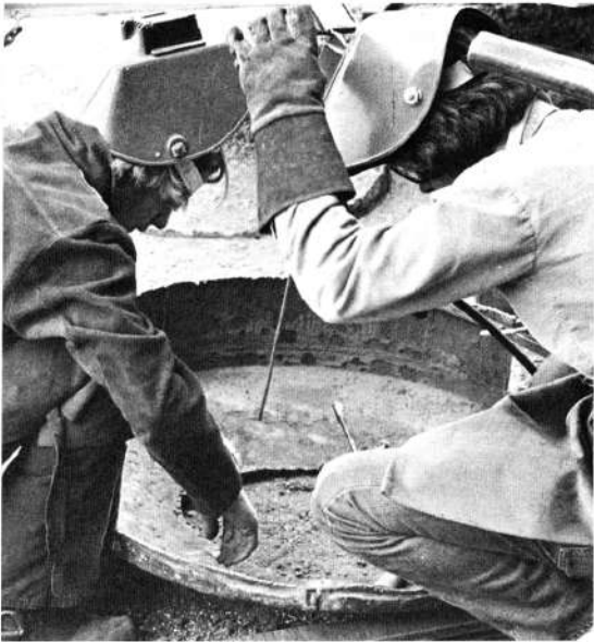
Robert Clayton and Don Alexander try to find out what happened while they were welding.
