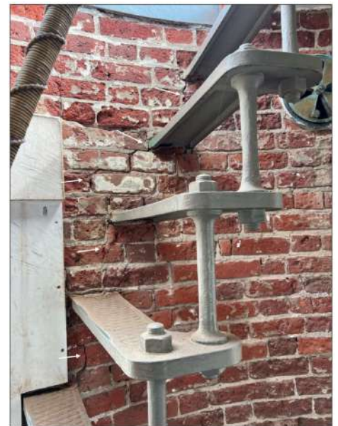
Extensive masonry cracking and crushing at embedded stair treads.
