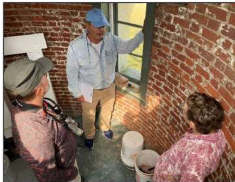
Pioneer Waterproofing removing interior wythes of brick masonry as required for inspection in the Cape Blanco Lighthouse Watch Room.
