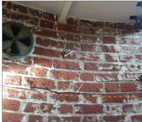
Vertical anchor wall crack meets horizontal window anchor wall crack.
